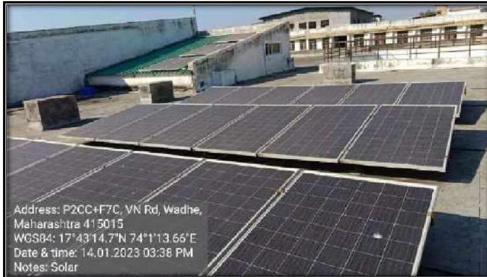
Fig. 7.1.3.9. Solar Energy Panel
